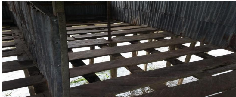
Fig. 1a. Floor wooden platform of the community toilet in the Sombrero river showing openings for faeces droppings into the river beneath
