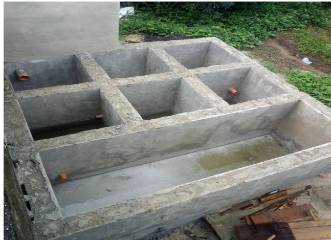
Fig. 5. Aerial view of empty treatment chambers of ESTS
