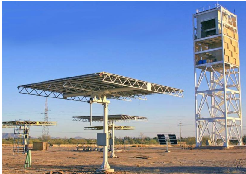
Fig. 1. Experimental thermo-solar plant in Sonora, México [16]
